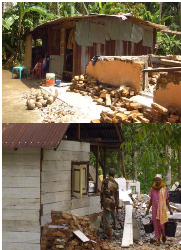
Community resiliency: Coping with the situation of houses severely damaged by the earthquake, families are rebuilding their own homes from salvaged materials and waiting for help.
