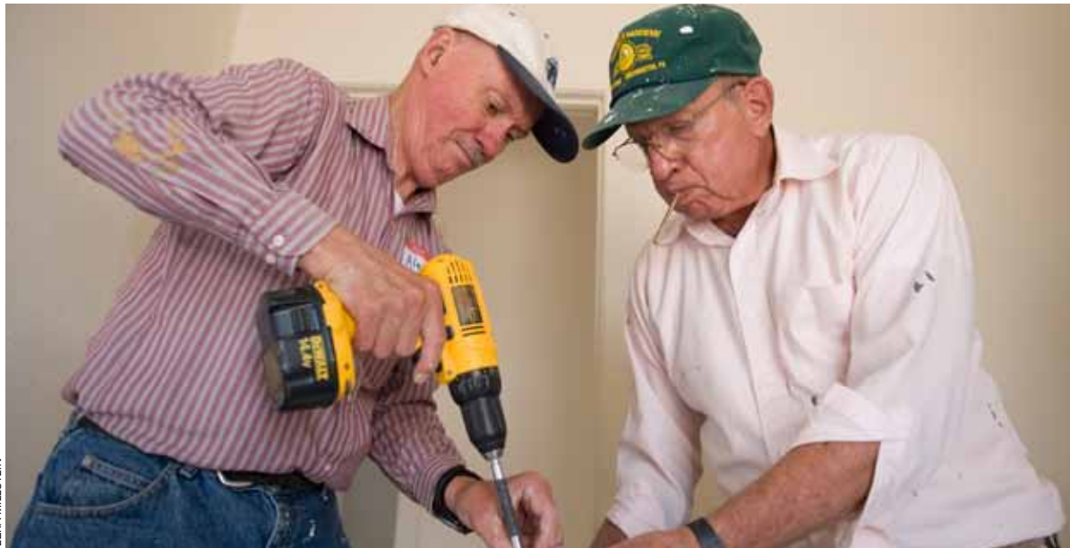
Volunteers Alex Zimmerman (left) and Hal Arner from Albuquerque, N.M., install a door in a new Habitat home.
