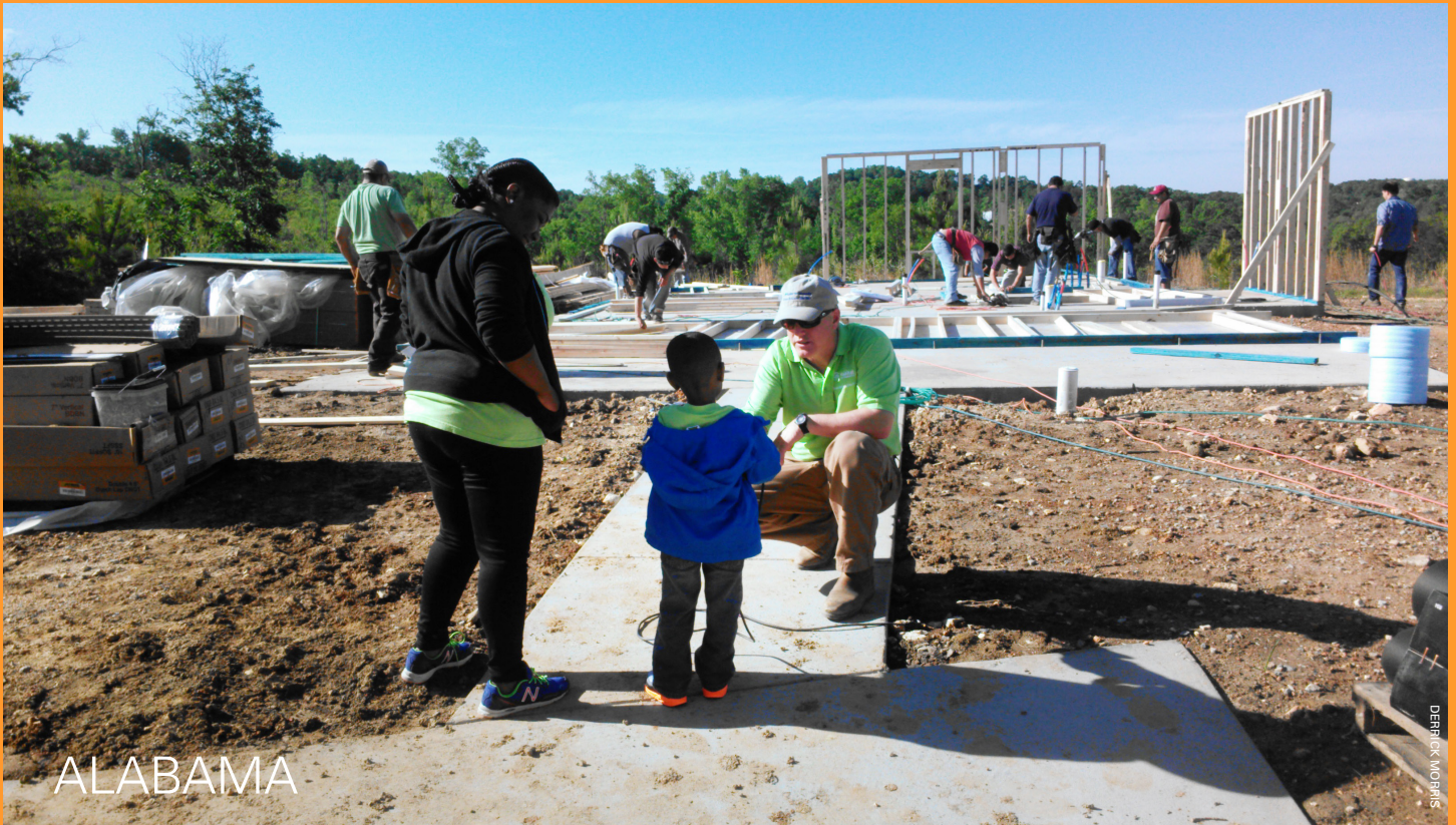
Alabama homebuilder Taylor Burton chats with Mentae Swanson at the site of the home where the boy and his mother, Oneasha Swanson, will live. The home was built in five days during Home Builders Blitz 2014.
