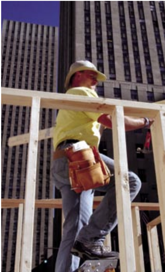
Erik Cullen of Seattle, Wash., joined other volunteers in New York City's Rockefeller Plaza to help frame houses for families affected by Hurricane Katrina. The Rockefeller Plaza build was part of Habitat for Humanity's Operation Home Delivery initiative and was featured on NBC's "Today" morning show.
