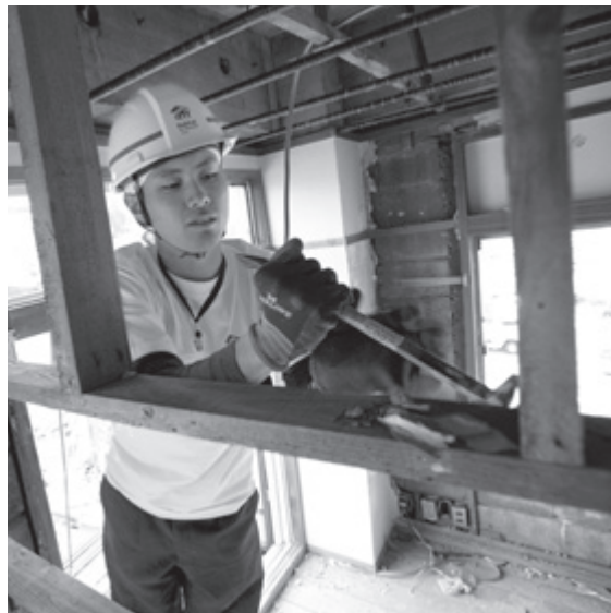
Habitat for Humanity volunteer Daisuke Kaneko works on the wood framing of a hotel in Rikuzentakata that was heavily damaged in the March 2011 tsunami.
