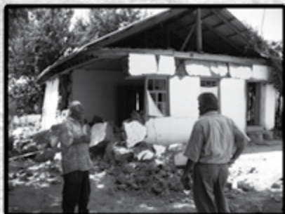
A homeowner surveys the damage of a 2006 earthquake in Kumsangir.
