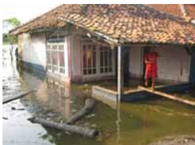
Home damaged by Karawang floods.
