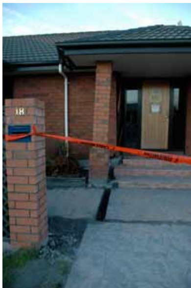
A damaged house after the earthquake.
